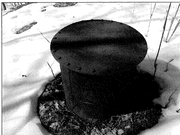
Access Manhole Cover Bolted to the Frames
