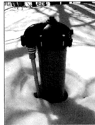
Well 3 lacking level instrumentation and labeling
