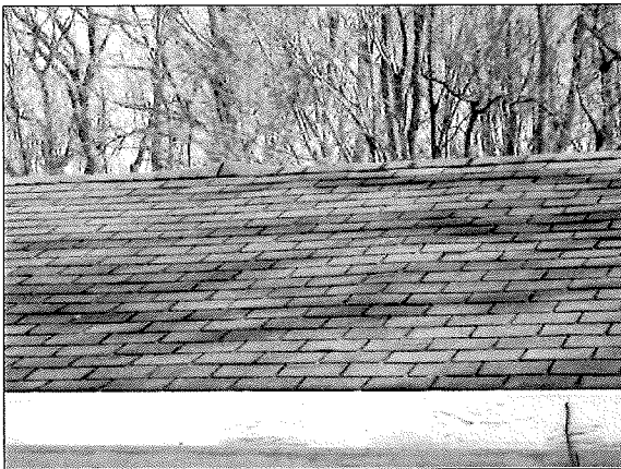
Deteriorated Asphalt Shingle Roof
