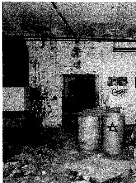
^ Debris and deterioration on the south building
